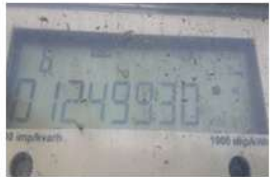
Figure 2. Electric Meter Image
