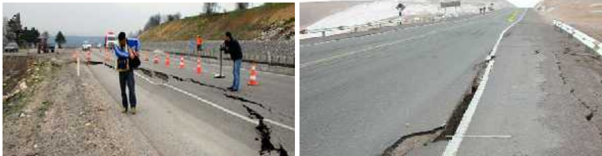
Figure 1. Highway settlements and shear deformations observed in Turkey (first one is from D-100 Highway stanbul-Ankara Direction , near Abant Intersection)
